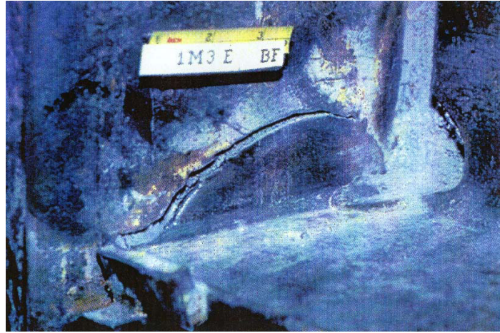
(a) “Divot” pull-out of column flange base metal.
